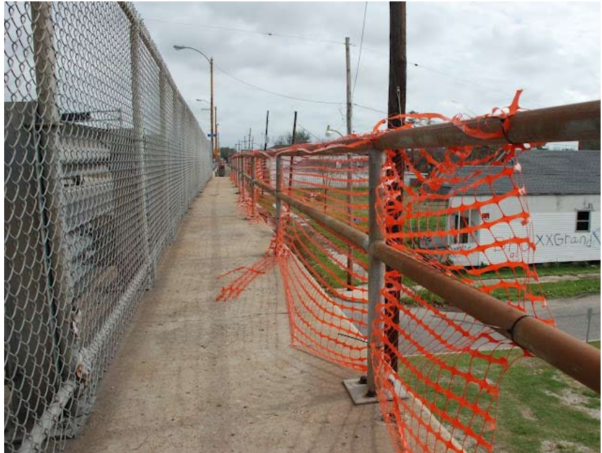
Figure 7: Orange plastic fencing was installed as a temporary measure on bridge railings to prevent accidents. Photo courtesy of Ct9.
