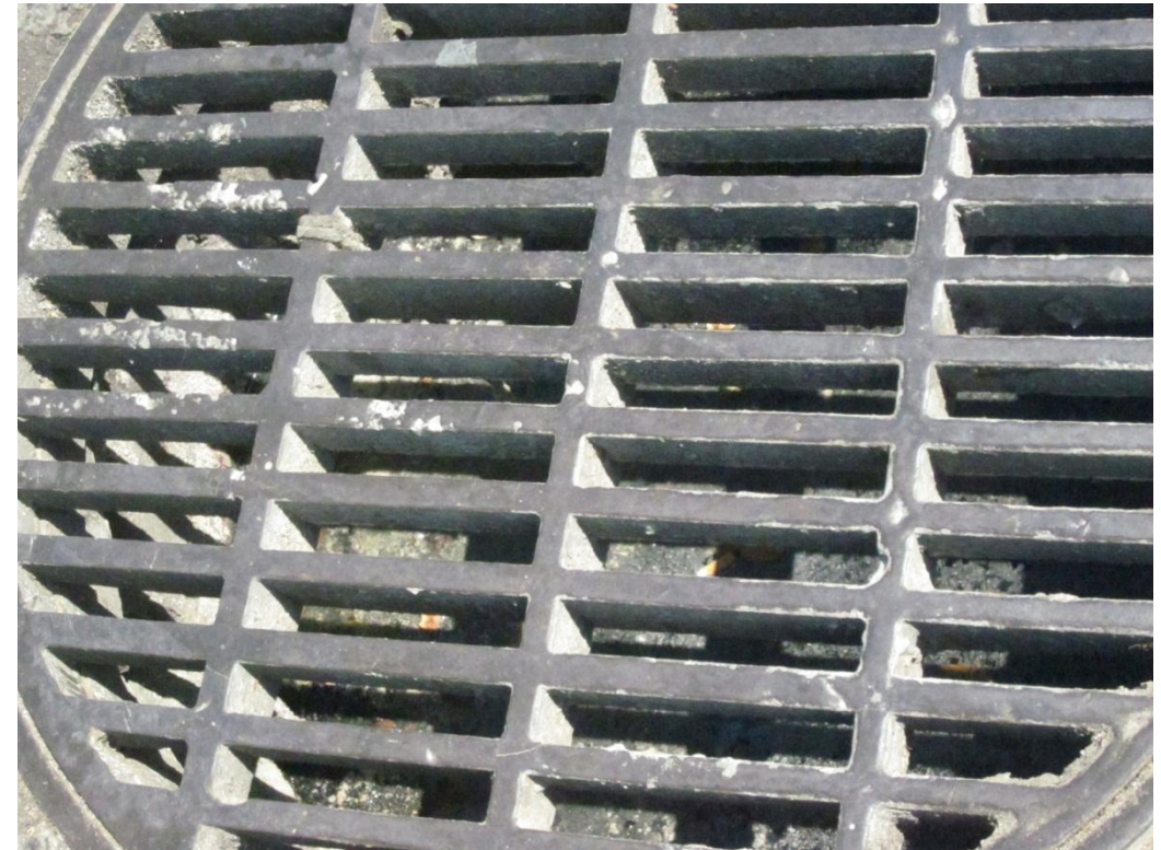
UNO Stormwater Inlet
