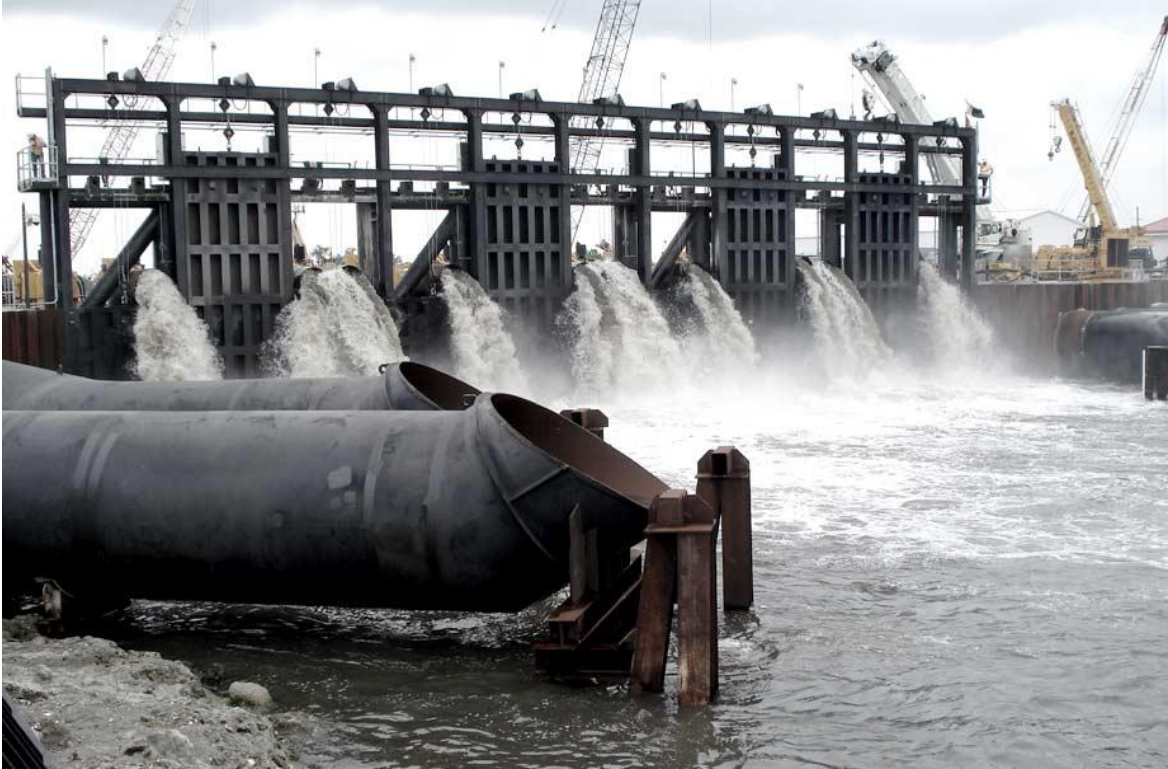
Photo courtesy of Gresham Smith and Partners
