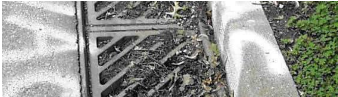
Example of a Clogged Drain. Source: http://www.msdcg.org
