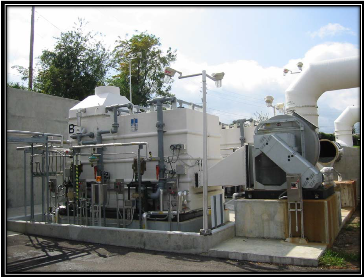
Figure 32: Odor Control System located at East Bank wastewater treatment plant
