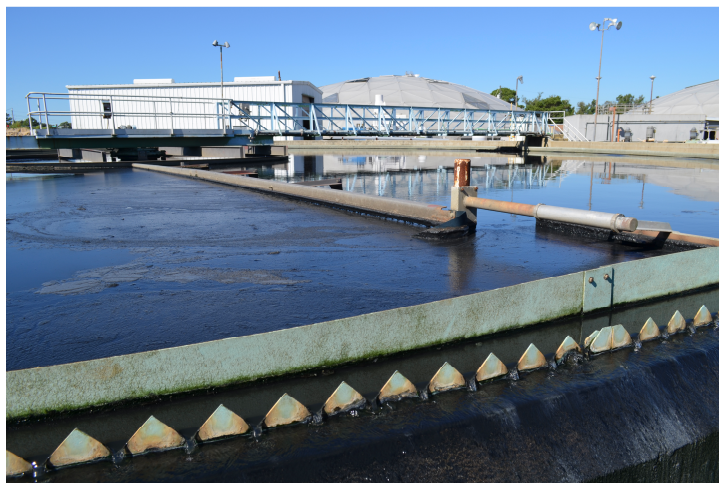
Figure 18. Wastewater flowing over the weir.
