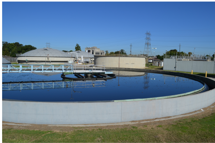
Figure 17. The secondary clarifier at the Marrero Wastewater Treatment Plant.
