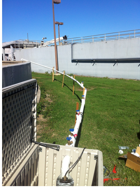
Figure 14. Continuous flow reactor at the Marrero Wastewater Treatment Plant.
